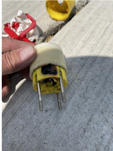
Above: photo showing your editor's shore power plug, I was investigating why my batteries were not charging and found that a weak connection in this end had been loose, and the bad connection had caused the burning of the plastic. Please inspect your cords!
